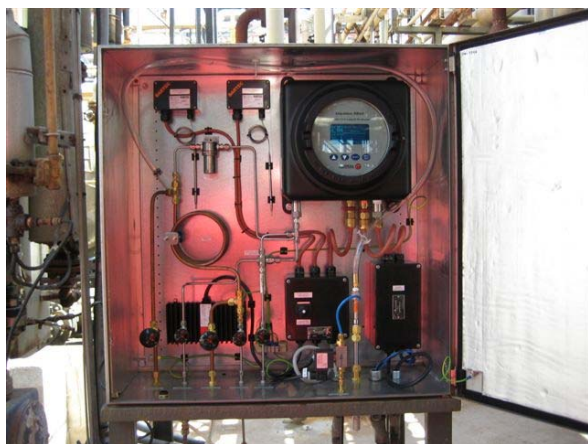
Liquidew EExd sampling system installed in process
