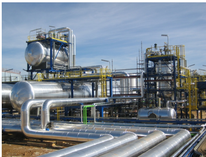
Moisture separation tank and condensers
